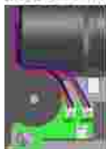
Battery connections on the front door
