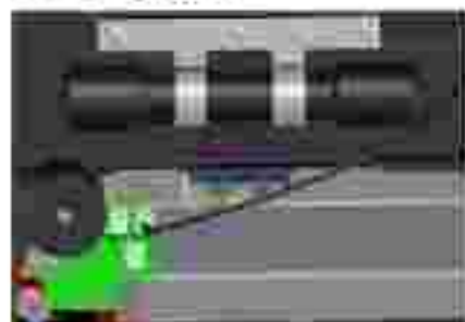
Fig. 24 Electrical backup battery
